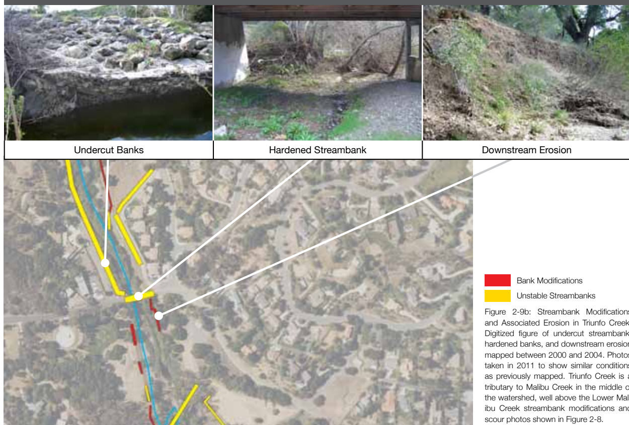
Figure 2-9b: Streambank Modifications and Associated Erosion in Triunfo Creek at Mulholland Highway
